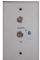
Antenna Power Supply
